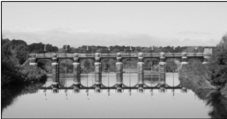
Dutton sluices, which were state of the art at the time of their construction in 1881.
